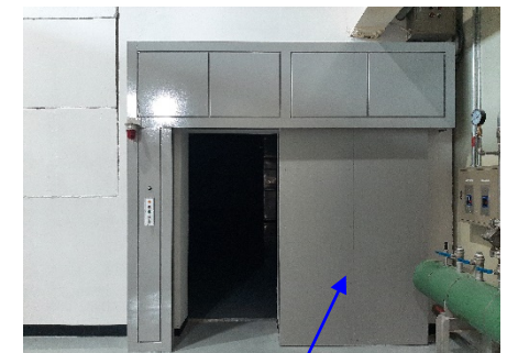
Sliding shielding door
