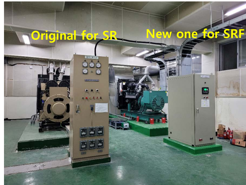
SRF-only Emergency generator
