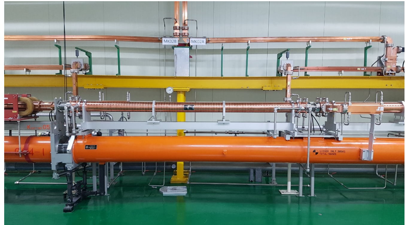
Newly installed accelerating column
